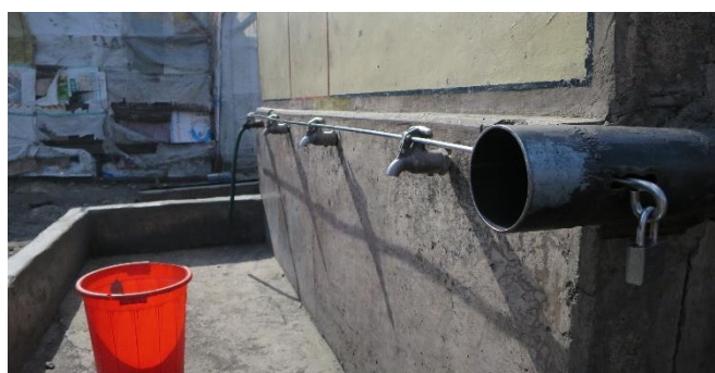
Closed taps in George Compound
